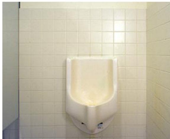
The ubiquitous waterless urinal, staple of green buildings, icon of fascination.
